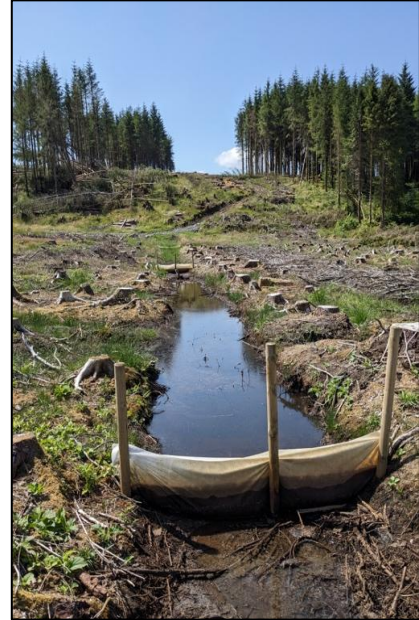
Figure 10: Silt trap for sediment control in a commercial forest.
